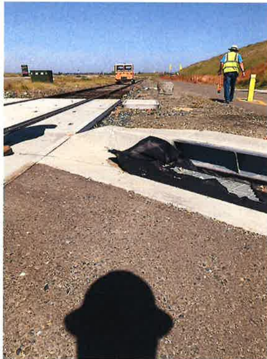
New crossings installed create multiple tripping hazards in the walkway (raised utility boxes, curb raised above sidewalks and roadway, crossing pads not filled in with ballast, and large rocks)
